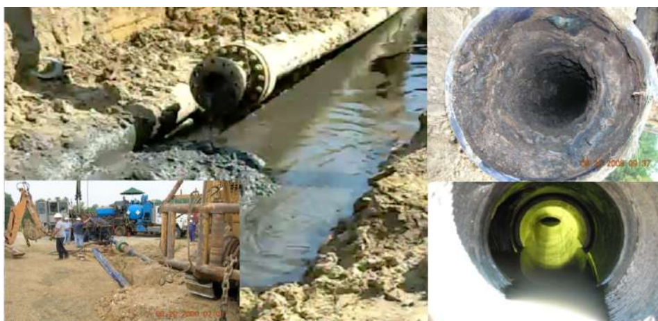
Figure 3: TFO Treatment for 10" Injection Flowline with Barium Sulphate Scaled Up, Illinois USA, 2008
